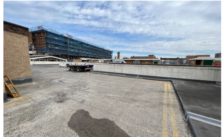
Above (left) door to/from first floor storage to loading area. (right) loading area.
